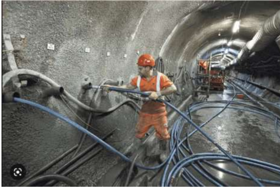
Fig. IV-8: Tunnel field leak injection (image source: Civillenggbliitz Website)
